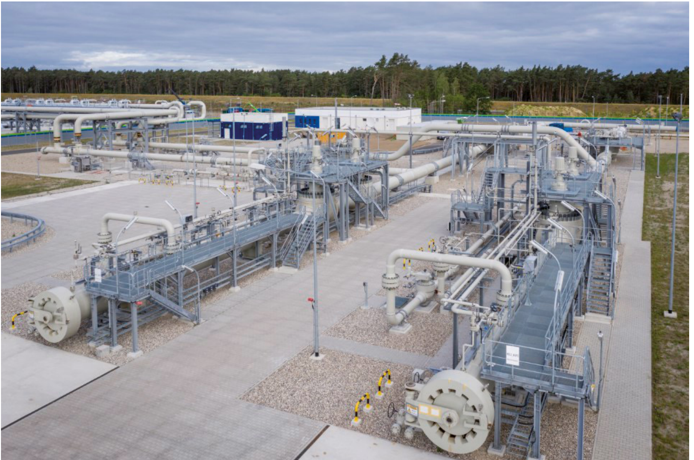
The pipeline inspection gauge (PIG) receiving station for the Nord Stream 2 Pipeline has been operational since the end of 2019. All necessary preparations for commissioning have been completed.
