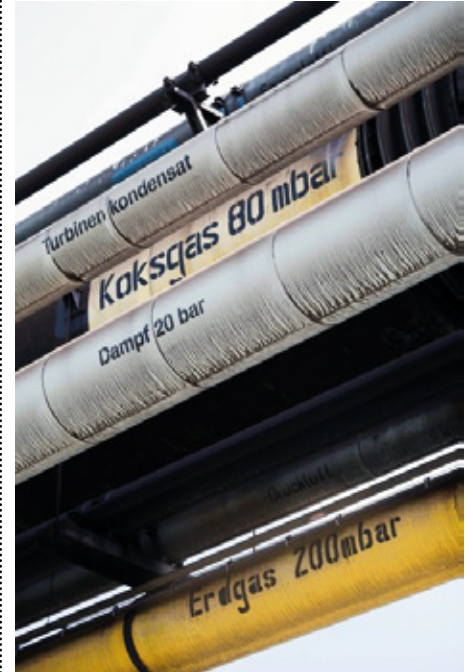
Existing pipelines can be used to transport the hydrogen from the PEM plant to the neighbouring galvanising plant.
