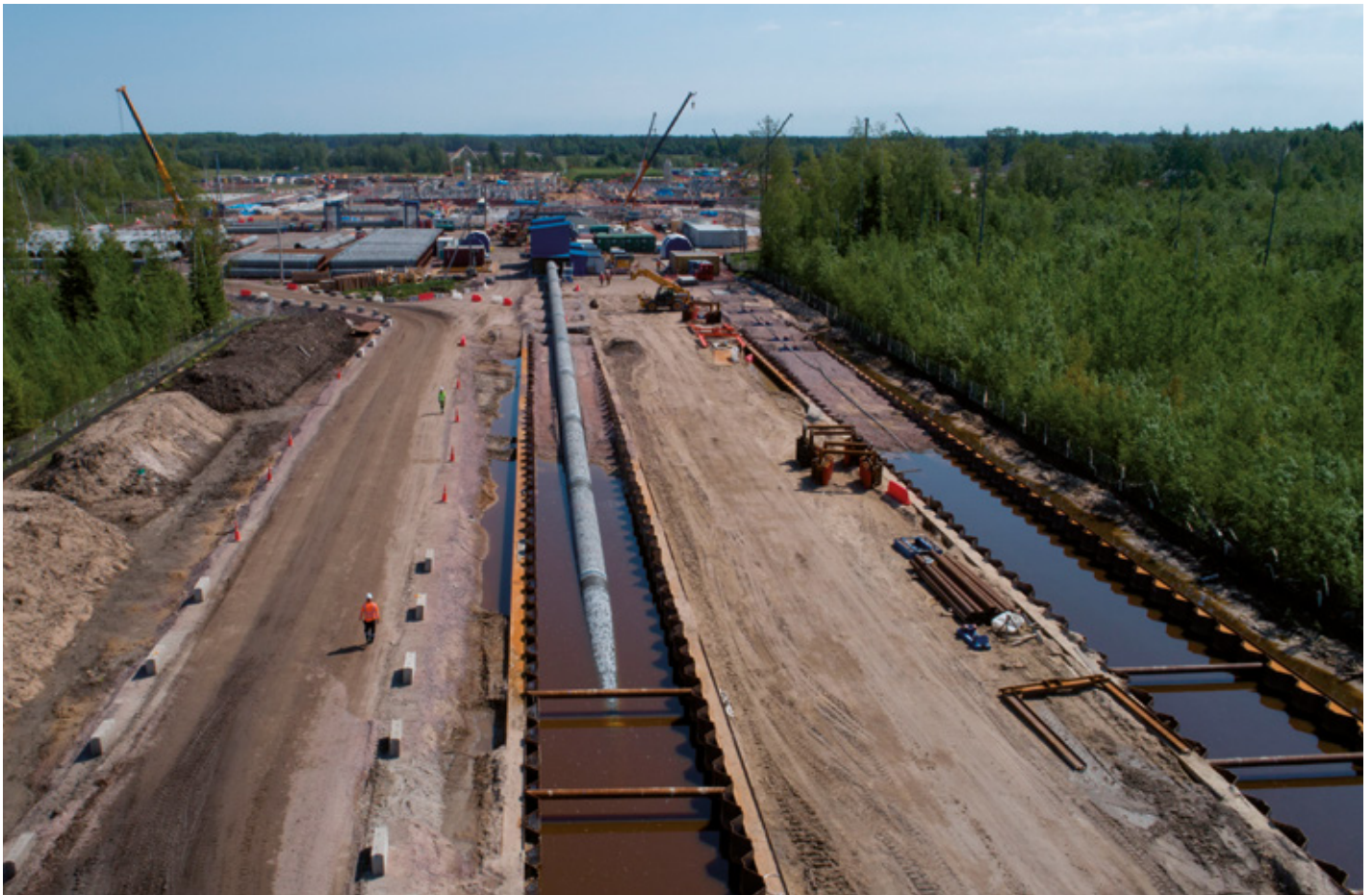
Pipe segments are welded together and pulled by a high-performance winch through water-filled trenches to connect the offshore Nord Stream 2 Pipeline with the Russian landfall facilities.
