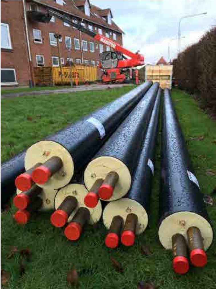
Storage of twin pipes (DN 50 Series 3 - Logstor) and building under renovation in Horsens, Denmark. | Image by Luis Sánchez-García
