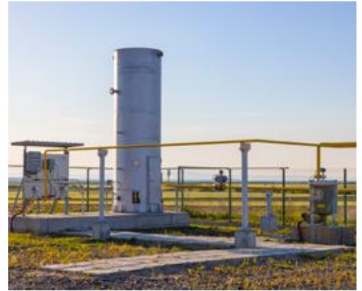
1 st photo – Moftinu Gas Plant - Enclosed Flare System
