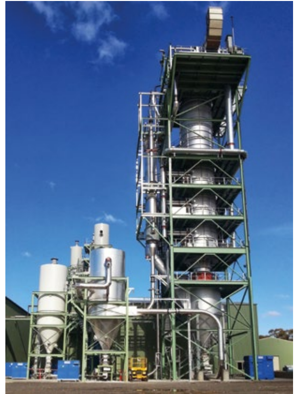
LEILAC 1 Pilot plant at the HeidelbergCement plant in Lixhe, Belgium
