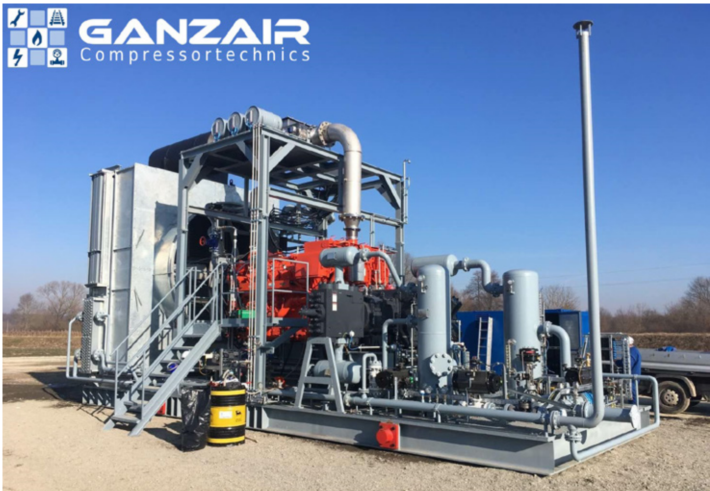
The equipment shown in the picture is a gas engine driven natural gas reinjection unit. Its function is to increase the layer pressure of oil wells for higher oil yield.
